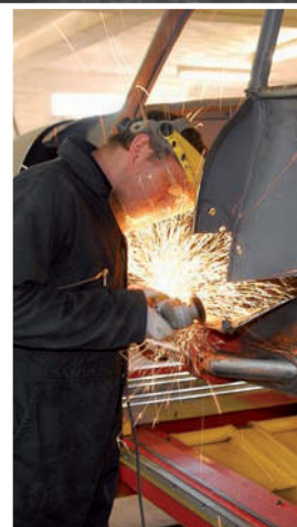
The company often welds in repair patches rather than fitting complete new panels to preserve as much originality as possible
